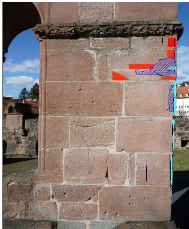
Figure 8: Eastern pylon with damage of resonance sound detector (red) and damage detection by IRT (hatched blue).
