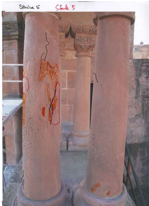
Figure 4: Pillar 5 (left), previous damage mapping, suspicion of subsurface detachment areas.
