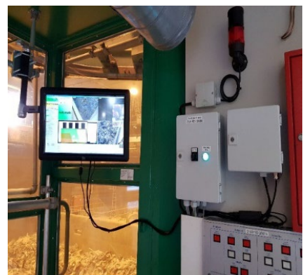
Fig. 4: Monitoring in the crane cockpit and alarm unit
