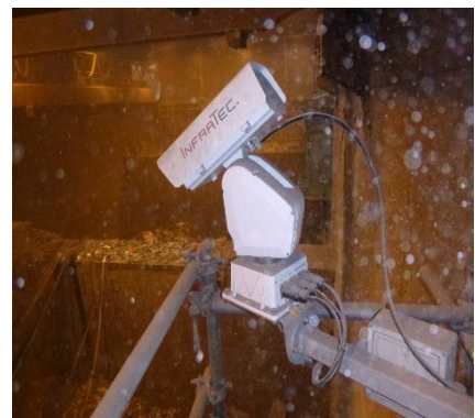
Fig. 3: TWIN system integrated in a very robust pan-tilt head in the waste bunker
