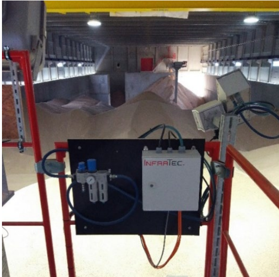
Fig. 1 The heart of the FIRE-SCAN hardware, well protected and equipped for continuous use
