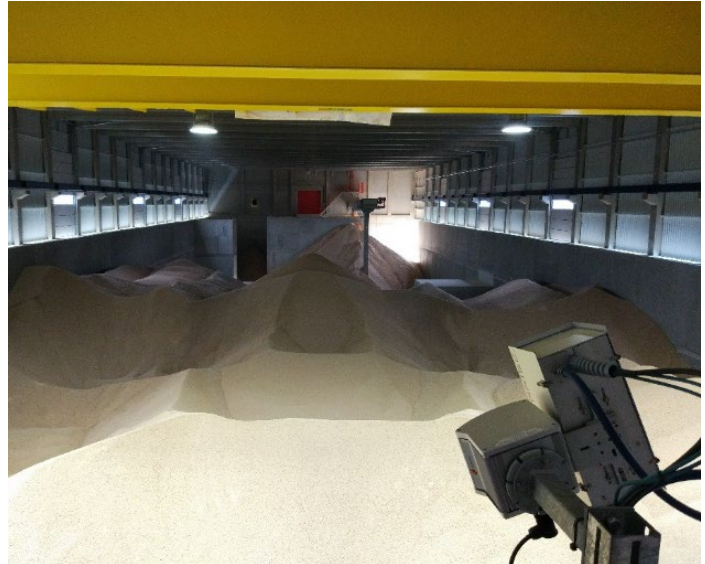
Fig. 2 A view into the pellet store, on the right the VarioCAM® HDx head on an automated pan-tilt head
