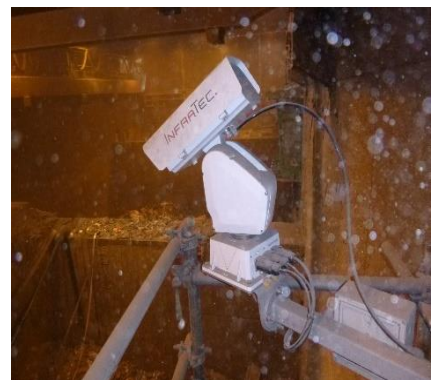
Fig. 3: TWIN system integrated in a very robust pan-tilt head in the waste bunker
